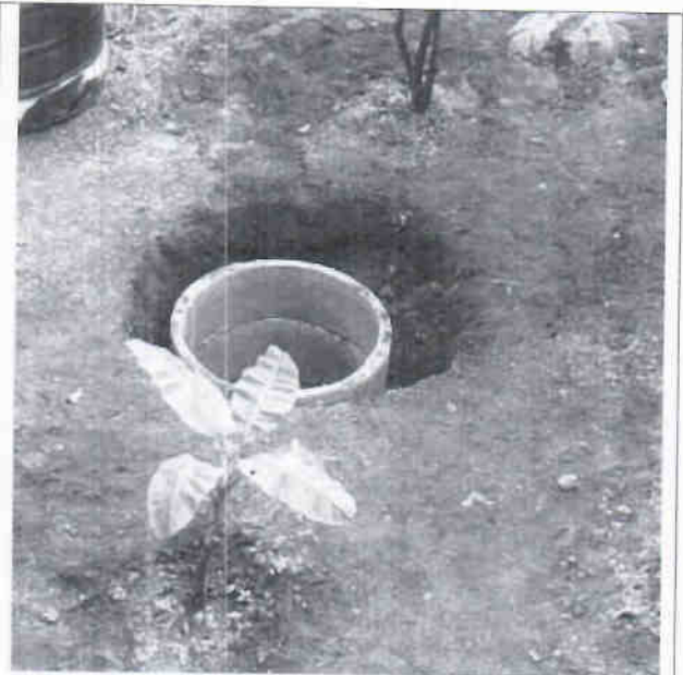
Percolation pit for rain water harvesting
